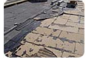
A few roof curbs and pipes eventually stopped this membrane from peeling across the field of the roof during Hurricane Charley. (Photo courtesy of RICOWI.)
