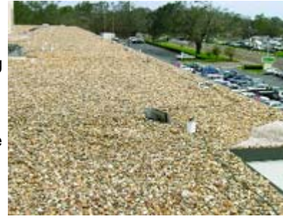
Gravel scour in right hand corner of ballasted roof after Hurricane Ivan. See the photo above for a close-up of the stone size used for this application.
