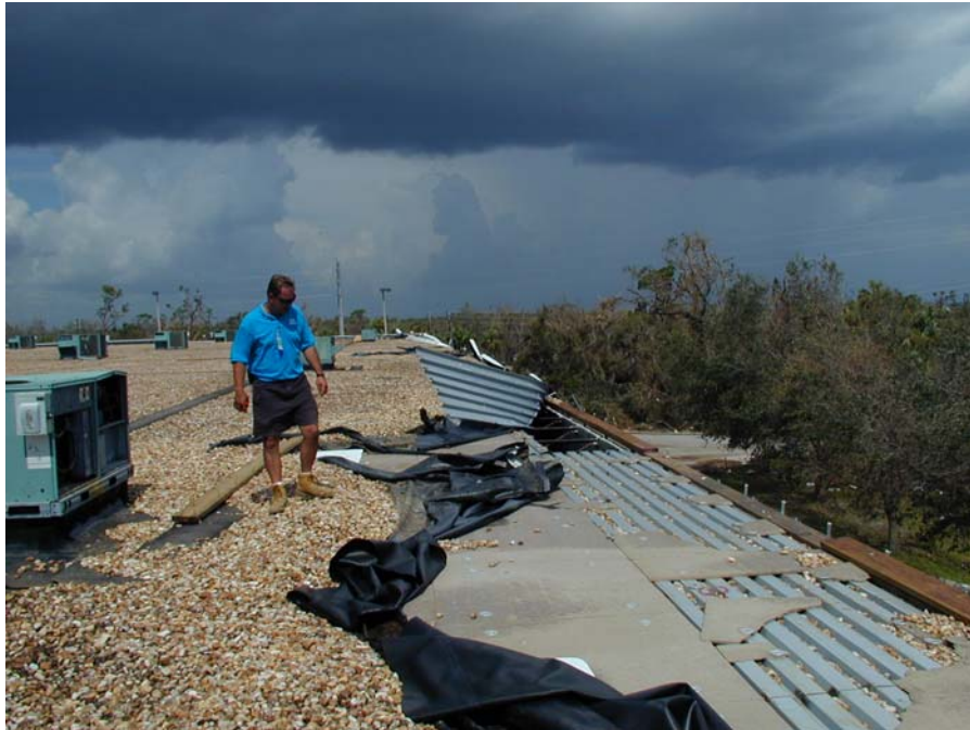
Figure 1 – Large retail building, Punta Gorda, FL, Hurricane Charley Photo courtesy of RICOWI
